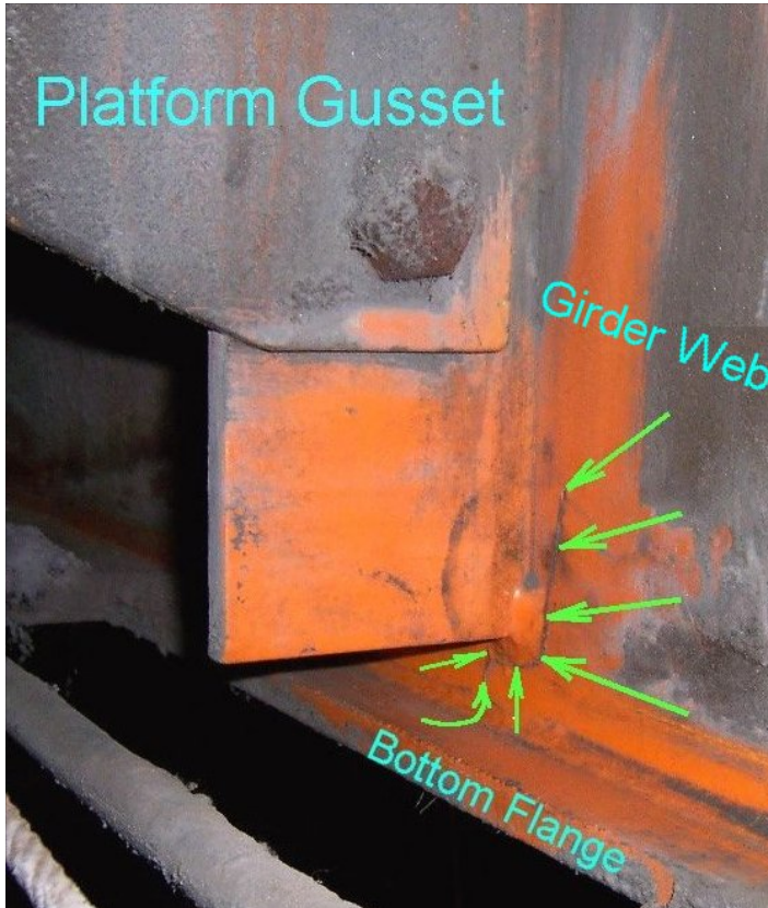
Figure 7-4 The girder web is cracked at the toe of the fillet weld for platform connection bar.
